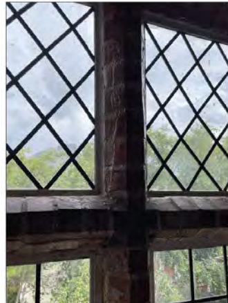
Figure 6B: Previously repaired cracking.
