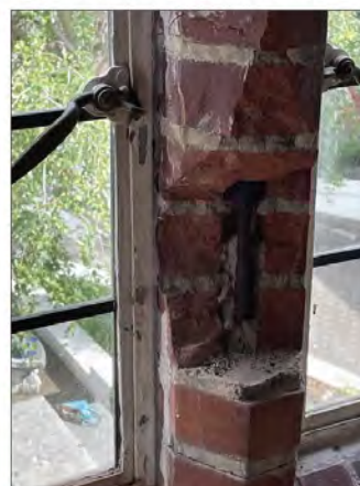
Figure 6G: Detail of spawling at vertical bricks.
