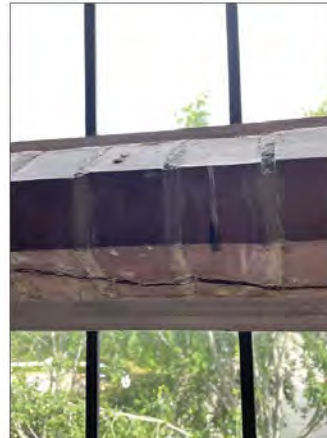
Figure 6C: Horizontal cracking in brick lintel.
