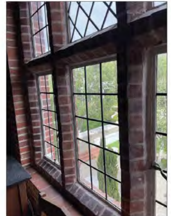
Figure 6D: Fine cracking in the brickwork.
